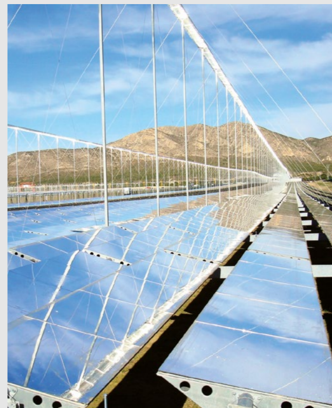
Photo Novatec – Puerto Errado 2
