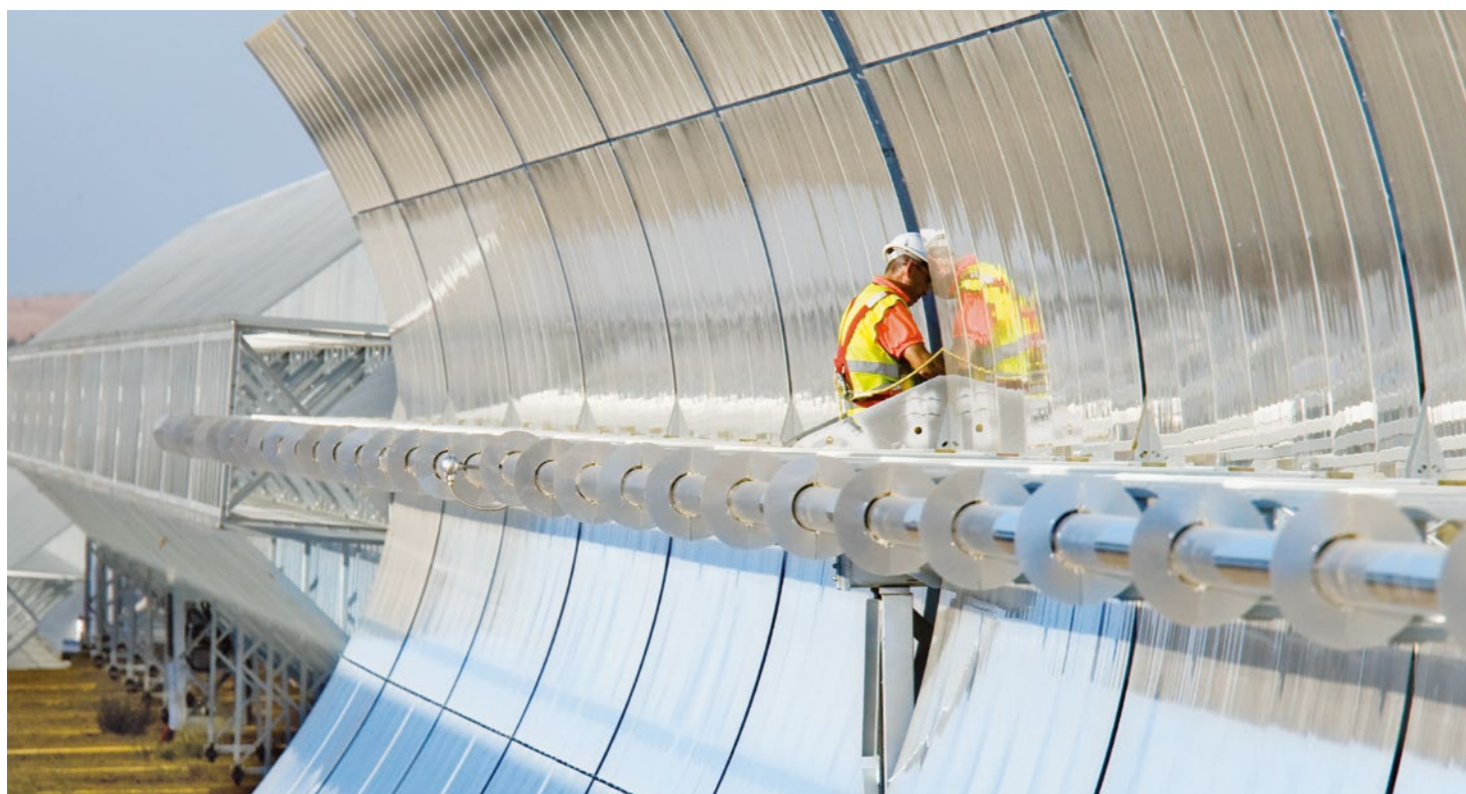
Photo ACS Cobra – Andasol 2
